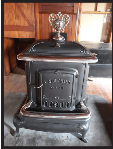
Our new, beautiful stove installed at the Town House
